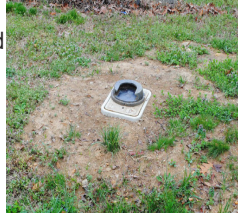
It's important to keep your gas and water meters clear of obstacles.
