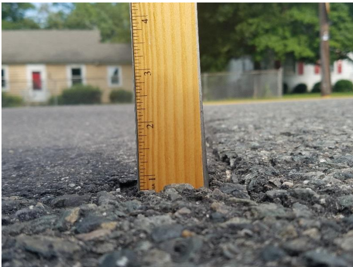
\frac{3}{4} inch deep at the corner of the repair made in February 2018.
