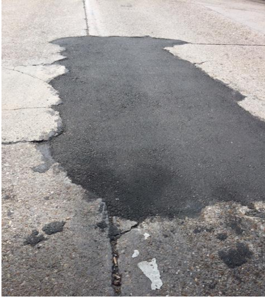
Concrete street restored with Asphalt, not squared.
