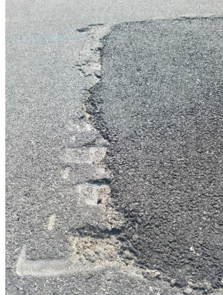
Marks from where temporary was dug up creating \frac{1}{4} inch dips in road.
