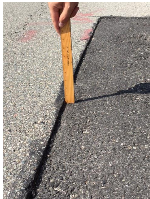
Not even with the road. Between \frac{1}{4} and \frac{1}{2} inch.
